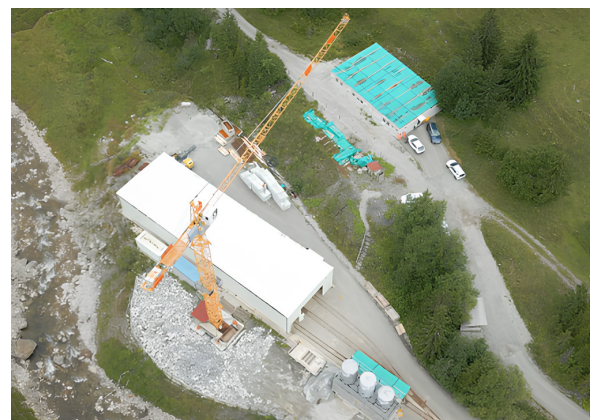
7 Aerial view of outdoor site installations
