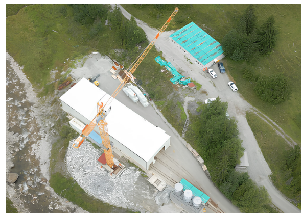
7 Aerial view of outdoor site installations
