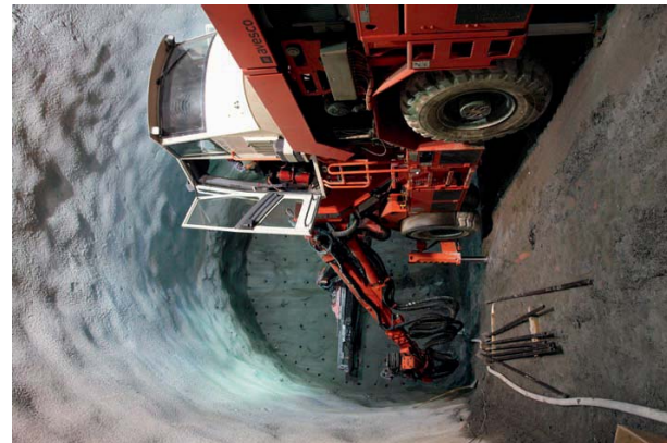
11 Anker in der Weströhre Nord Sigrino Rock bolting in the northern west bore, near Sigrino
