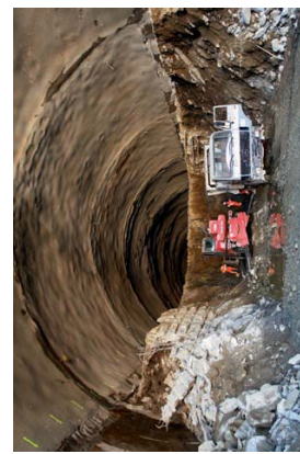
10 Portal Vezia: Strossabbau in der Kaveme Ost The Vezia portal: excavation of the bench in the East Cavern
